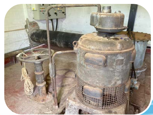
Langley Double redundant slip ring motor pump
