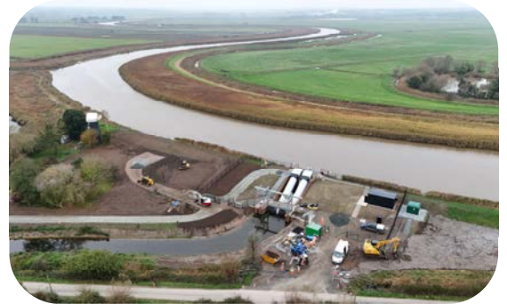
Aerial Image of the completed Norton Pumping Station. Photo Credit BAM UK
