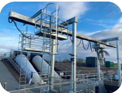
The Fish Friendly Archimedes Screw Pumps and the new Weed Screen system.
