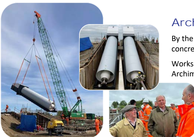
The Archimedes Screw Pumps arrive & The Board visit to see the project progress. Photo credits: WMA
