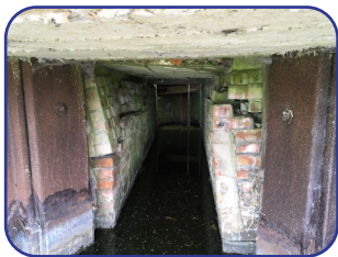
Short Dam Pumping Station Inlet
